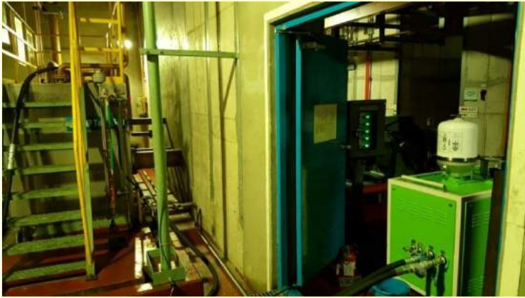
PCC602 Installation Hose Line
