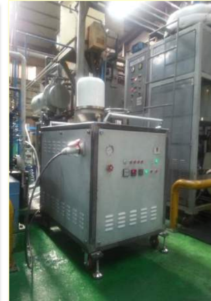
Dae Sung Heat treatment PCC602 installation
